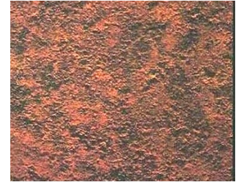
Condition D Unblasted
